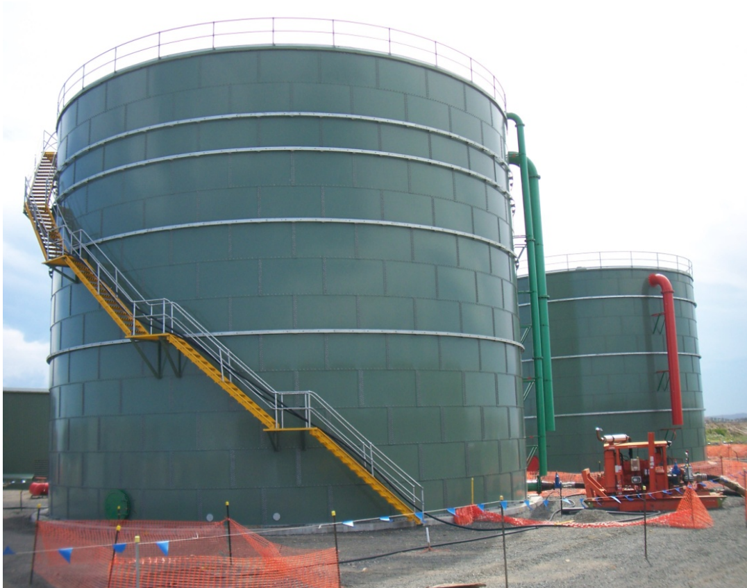
Figure 2.12: Water Storage Tanks
