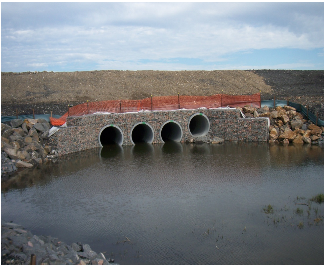
Figure 3.10.2: Installed Rail Culverts for Green and Golden Bell Frog Movement
