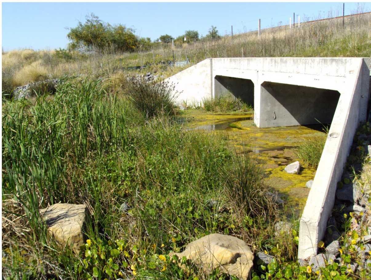
Figure 3.10.2: Amphibian underpass of rail infrastructure
