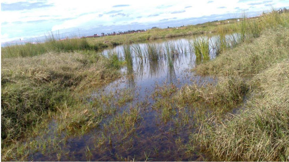
Figure 3. Localised flooding at Pond 15 as a result of frequent rainfall and high groundwater levels
