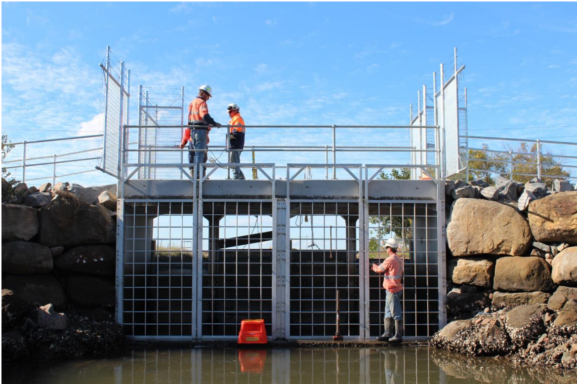
Plate 18: Installed MPED 2 screen (debris-style screens)
