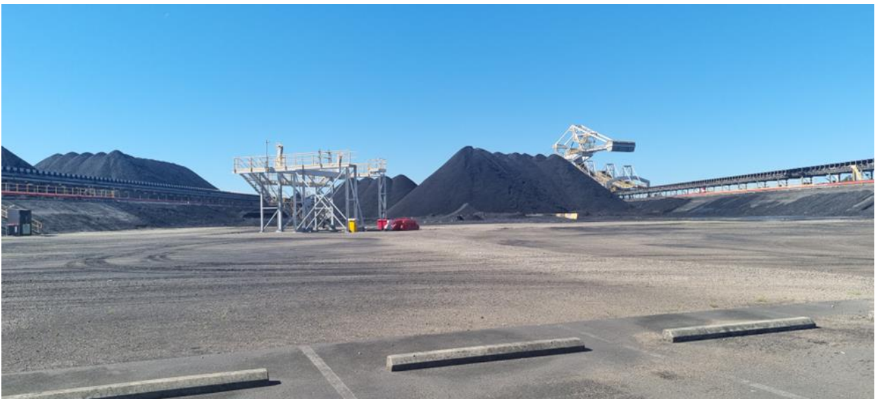
Photograph 4 – Stockpile area (photoground foreground) stabilised (veneered) with Vital Bon-Matt Stonewall (chemical dust binding agent).
